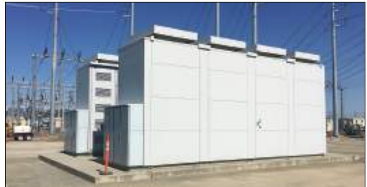
PG&E's Vaca-Dixon sodium-sulfur battery energy storage system charges batteries when demand is low and then sends reserved power to the grid when demand grows.
