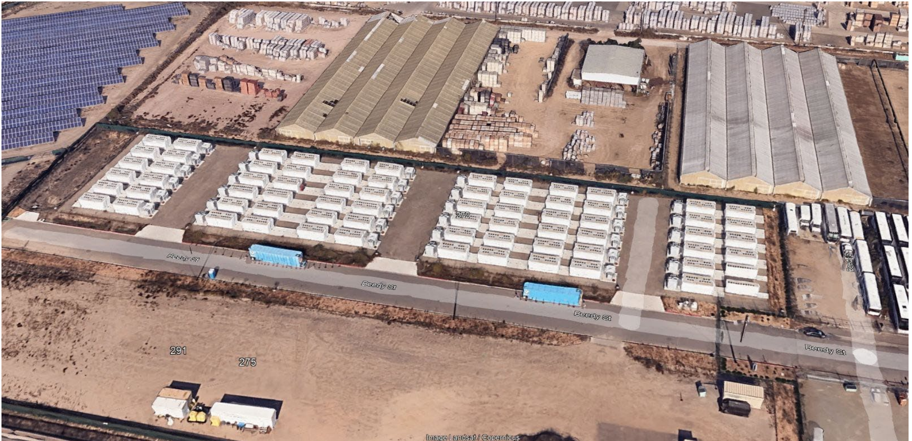
Oxnard Battery Storage Facility Beedy St just west of E. Vineyard Ave
