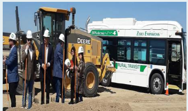
Dignitaries don hard hats and pick up their shovels to break ground
