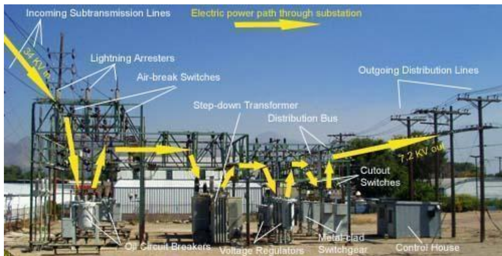
Typical Substation: https://www.osha.gov/etools/electric-power/illustrated-glossary/sub-station
